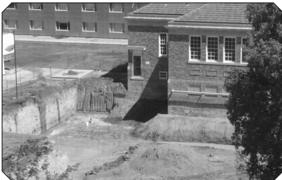
The Mari Sandoz Heritage Center under construction in 2001. Sandoz often expressed a hope for the development of an educational and cultural facility depicting the heritage of the region she called home.
